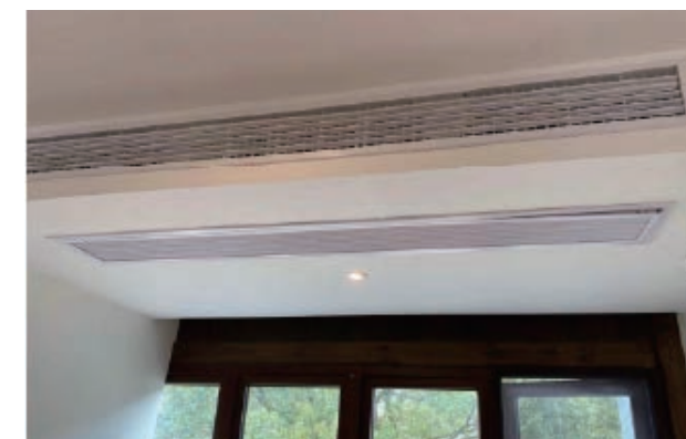
Figure 5-3-2-10 Exhaust air heat recovery unit
