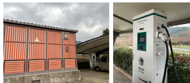
Figure 5-1-1-3 Charging and battery for electric cars
