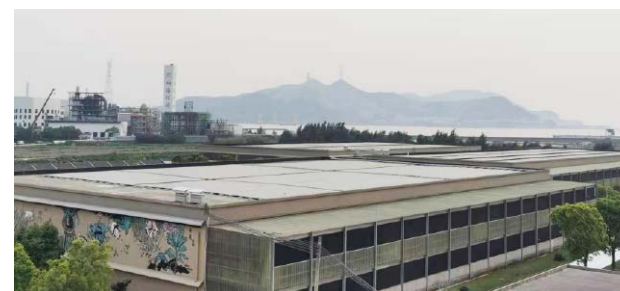
Figure 5-1-3-5 PV panel installed roof
