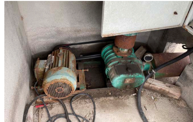
Figure 5-2-1-10 Oxygen supply equipment
