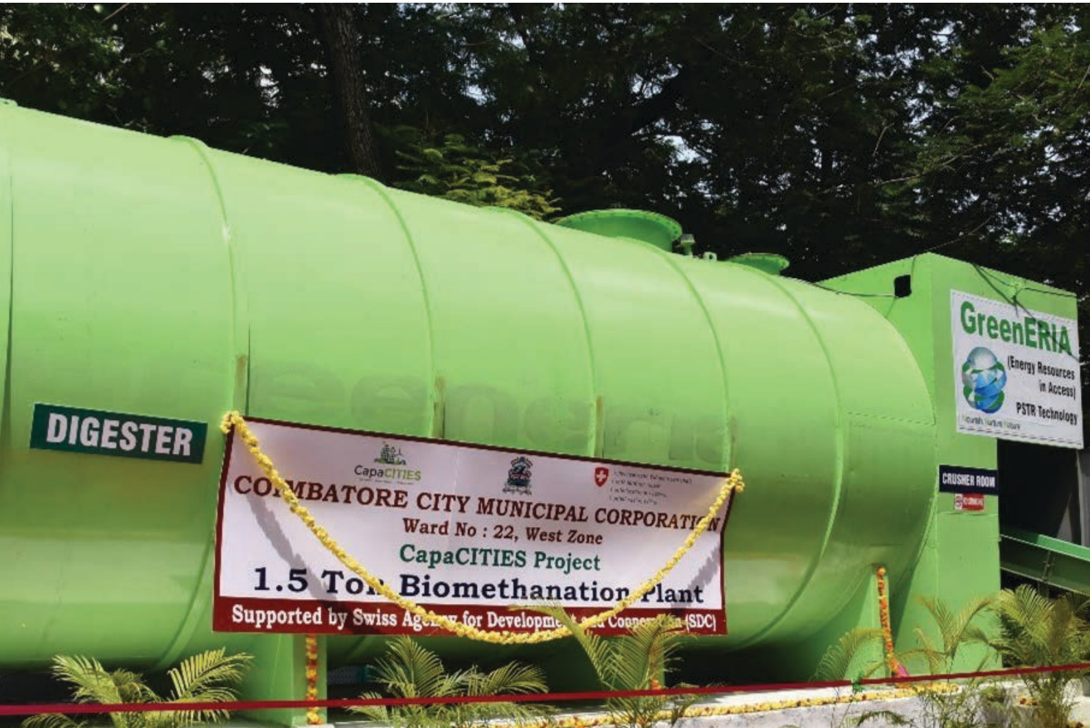
Image 21: The bio-methanation plant commissioned by Coimbatore Smart City produces approximately 60,000 m 3 of biogas and 39,055 m 3 of methane annually, generating around 7 KW of electricity per day. Source: Coimbatore Smart City.
