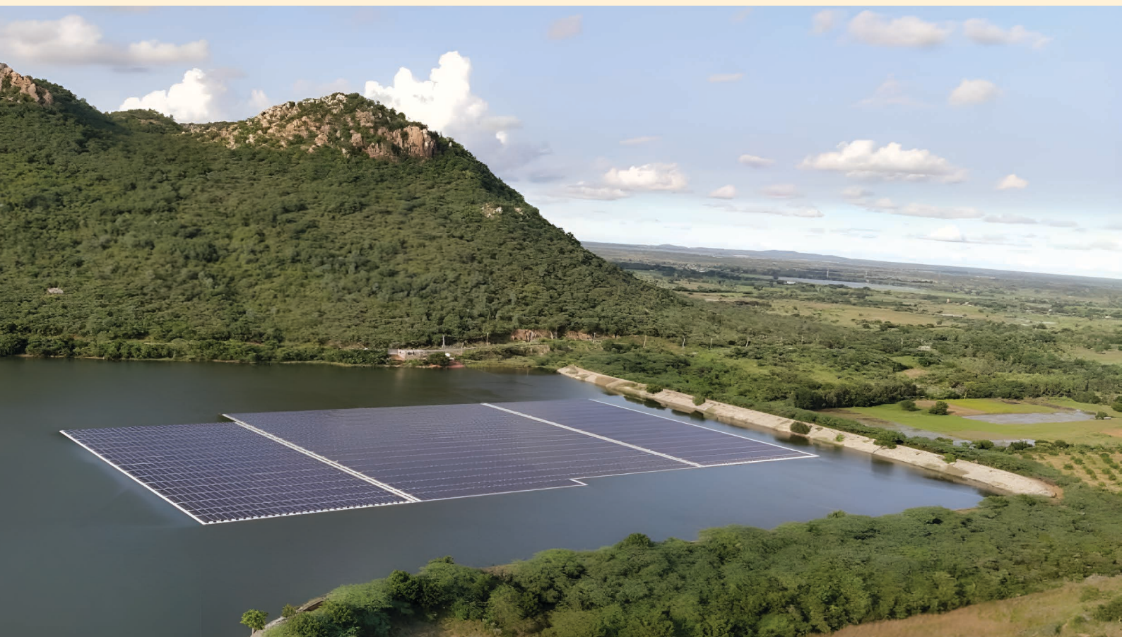
Image 19: A 4-megawatt floating solar plant commissioned as part of SCM in Tirupati (Andhra Pradesh). Source: Tirupati Smart City
