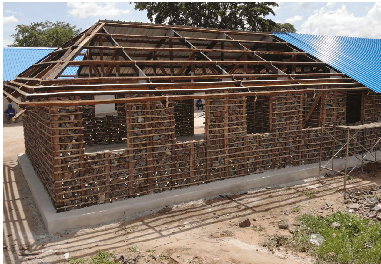
Complete Primary School in Mecutusse reconstructed with mixed materials under the ERRP Project | Source: UN-Habitat
