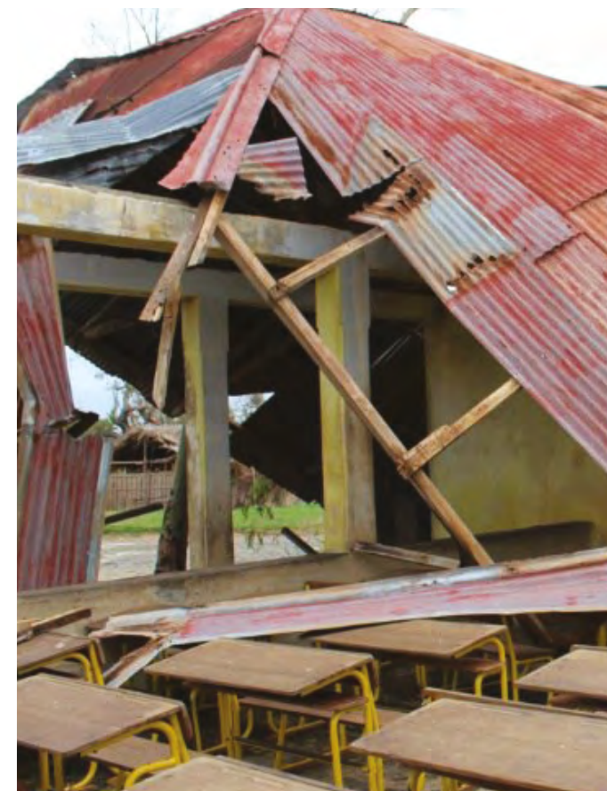
School damaged by Dineo Source: Earth Chronicles News earth-chronicles
