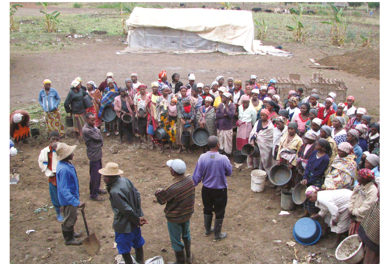
Participatory Construction of the Elevated School of Maniquenique, Gaza Province | Source: UN-Habitat
