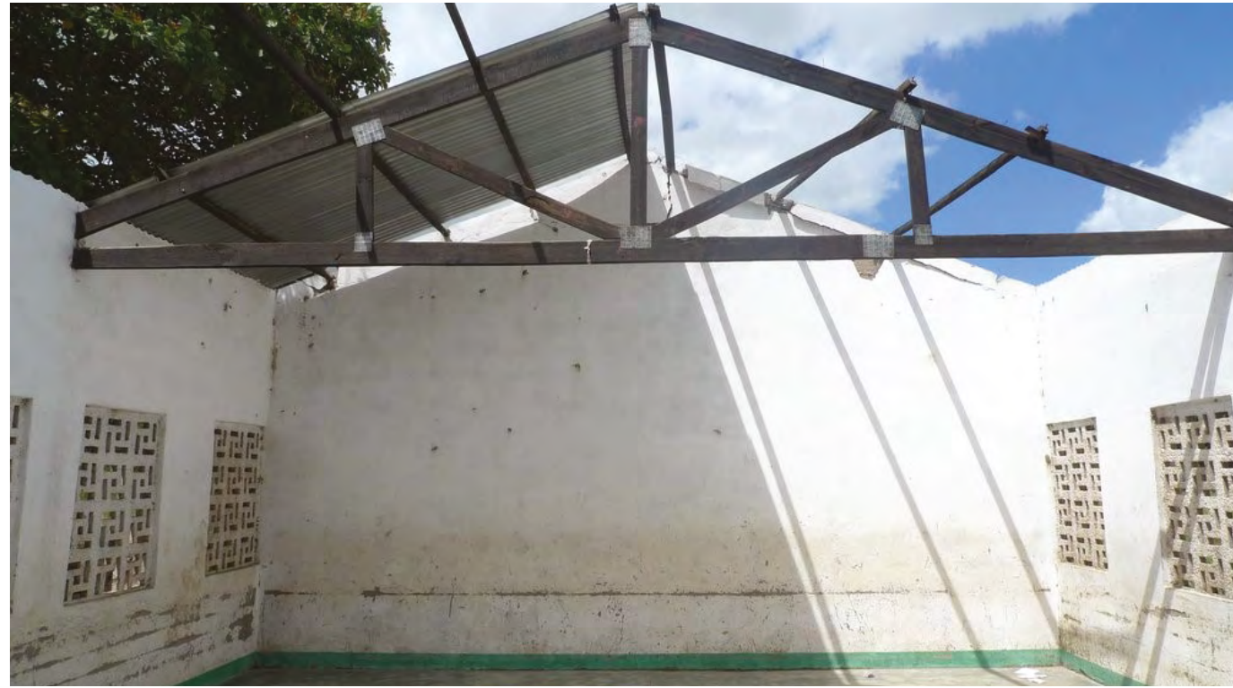
Damages at Nicoadala's school | Source: UN-Habitat
