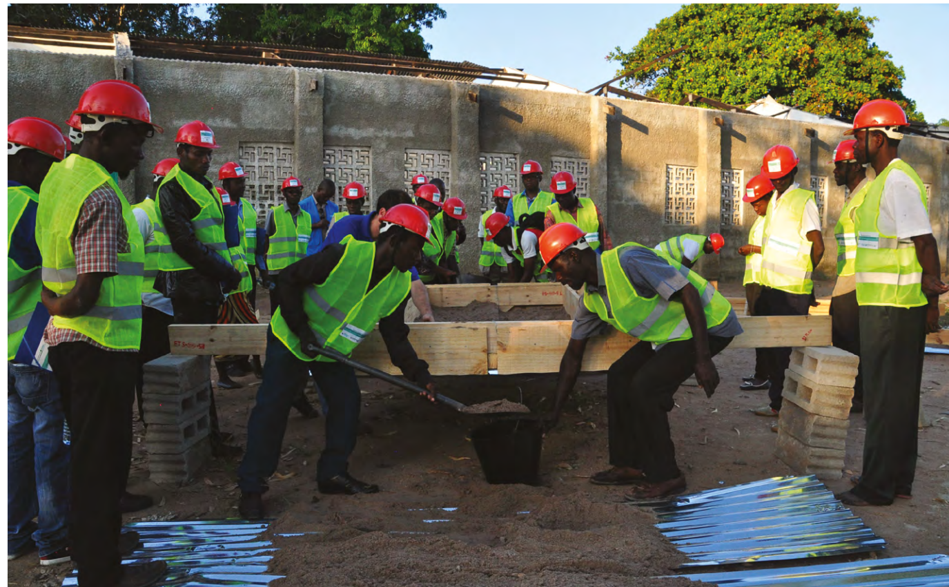
On the job Training in Resilient School Reconstruction in Nicoadala | Source: UN-Habitat
