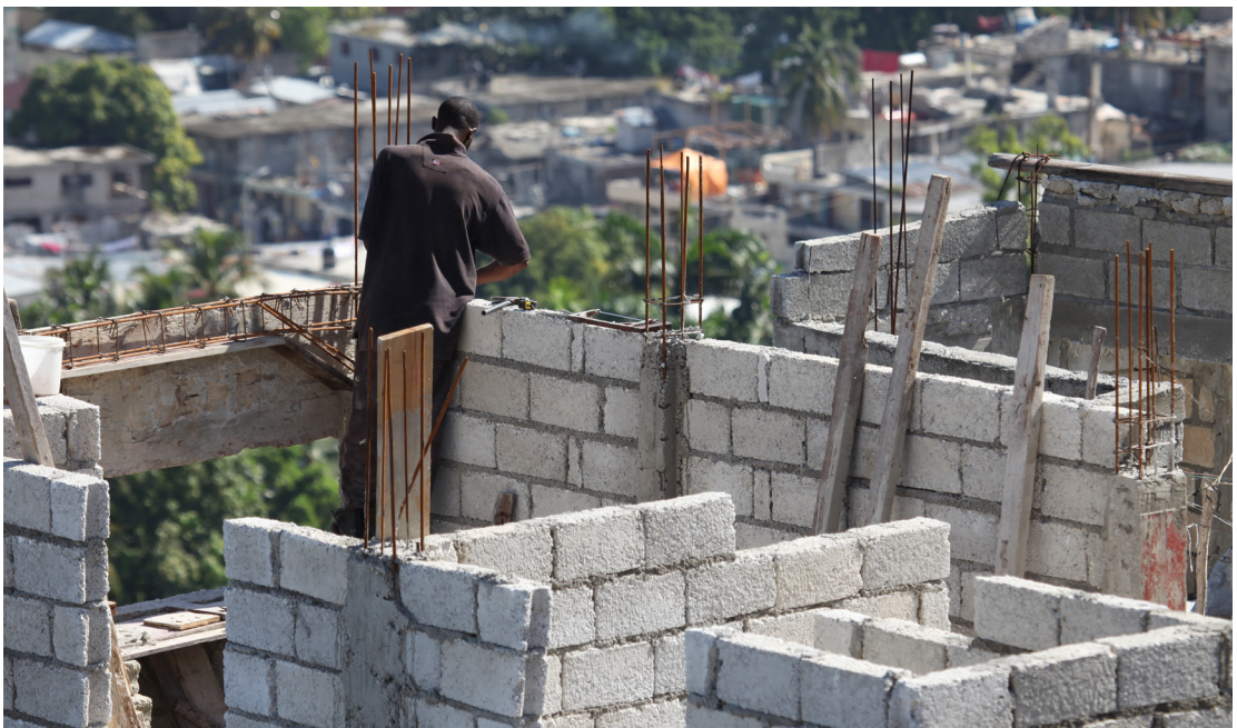
Ongoing construction in Port-au-Prince, Haiti. After a devastating earthquake struck the country © Julius Mwelu/UN-Habitat
