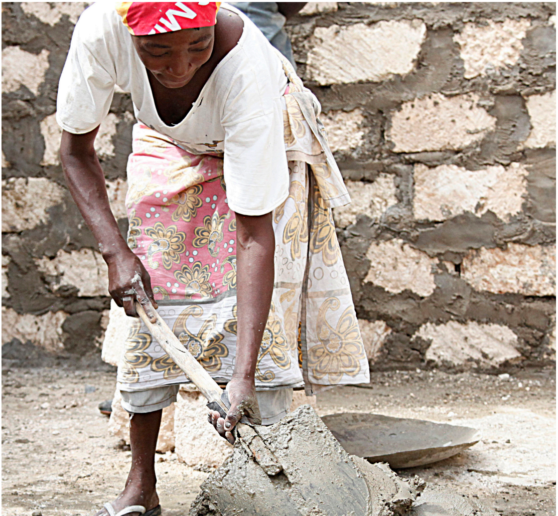
Ongoing construction of proposed Majengo Empowerment Centre in Kilifi, Kenya 2016 © Julius Mwelu/ UN-Habitat
