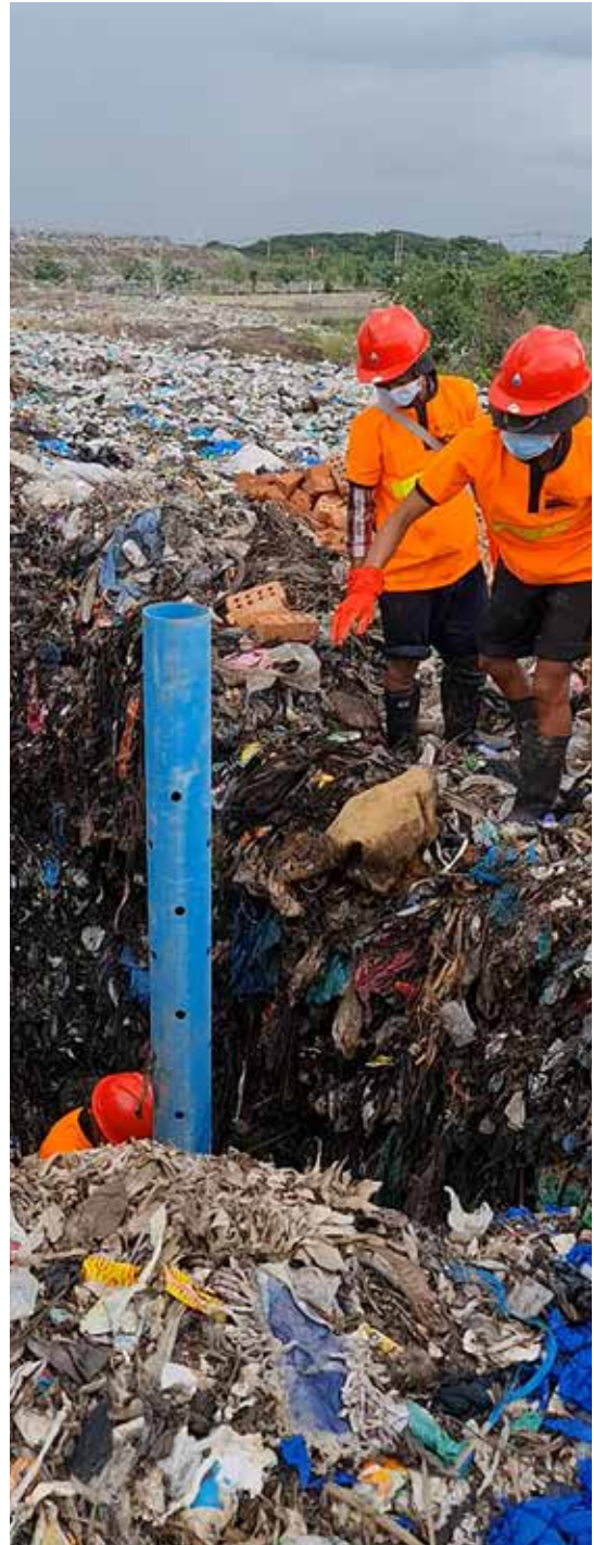
Installation of Fukuoka method perforated pipes at the Htein Bin FDS © UN-Habitat
