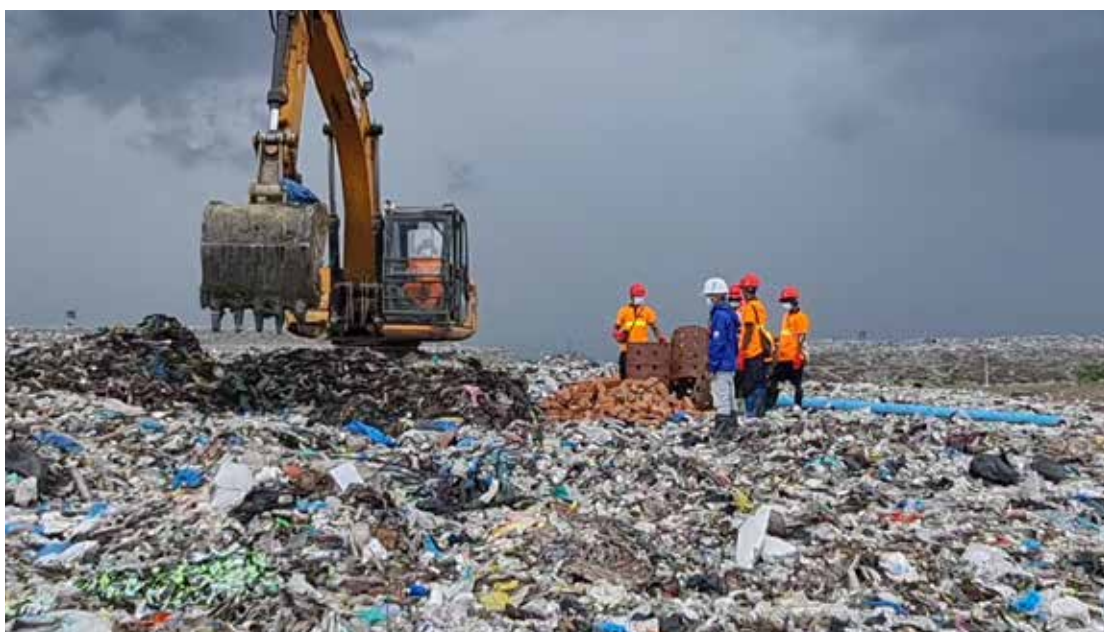
Installation of Fukuoka method perforated pipes at the Htein Bin FDS © UN-Habitat
