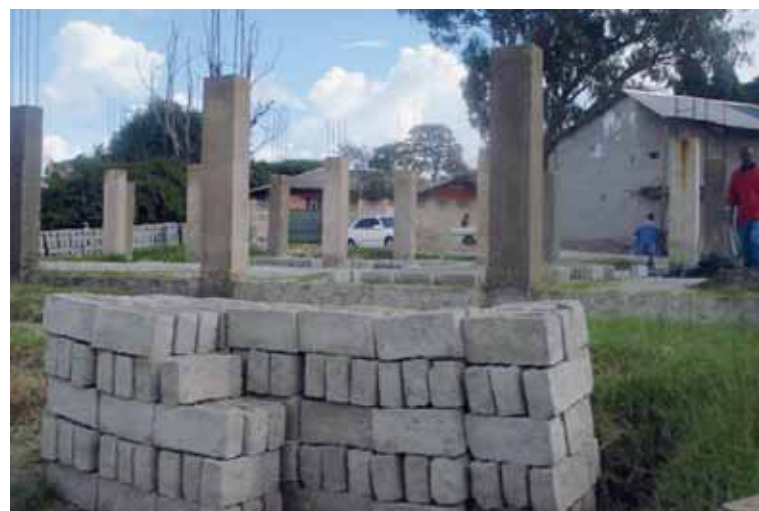
Figure 75. Informal construction with blocks and in situ concrete columns, Kitwe. Photo © UN-Habitat/Daniel Phiri
