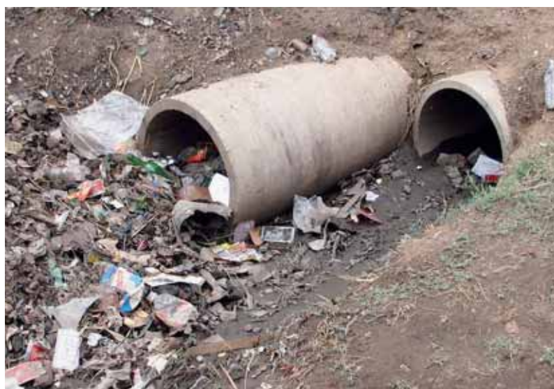
Figure 58. Garbage blocking a drain, Chaisa. Photo © UN-Habitat
