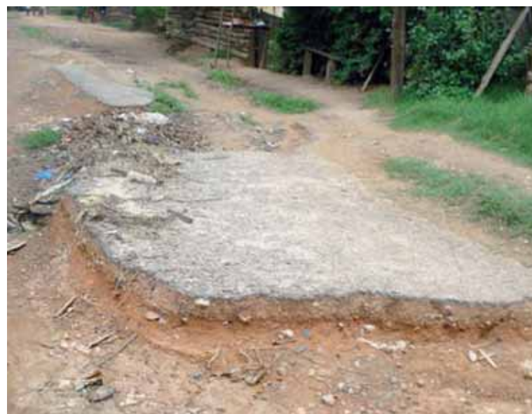
Figure 56. Broken tar road in Buchi, Kitwe. Photo © UN-Habitat
