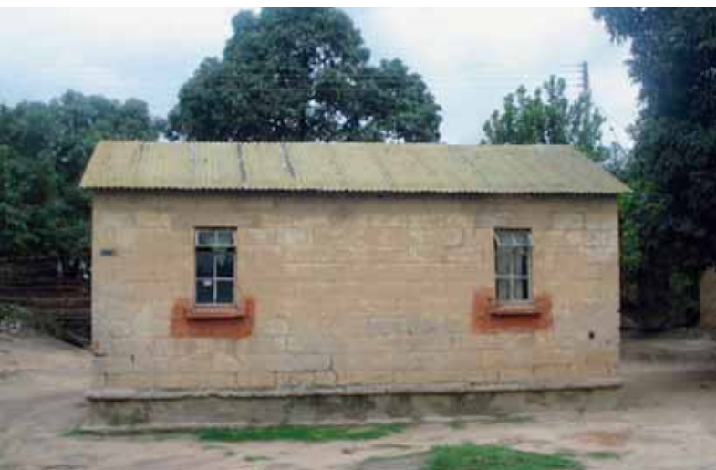
Figure 79. A stabilised soil dwelling over 60 years old, Buchi, Kitwe. Photo © UN-Habitat/Daniel Phiri
