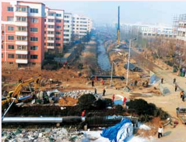
“11 • 22” Pipeline Leakage and Explosion Site, Qingdao (Photo by Yu Fangping)
