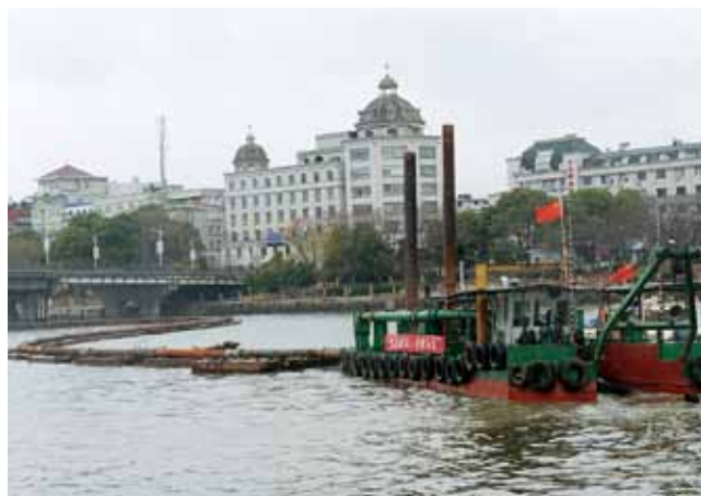
Dredging vessels are working on Yiwujiang River, Zhejiang Province on February 7, 2014 (Photo by Zhang Yunfei)
