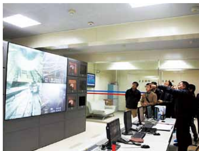
Comprehensive Utility Tunnel and Monitoring Center of Guangfu Road, Kunming (©/ Http://www.ynjst.gov.cn )
