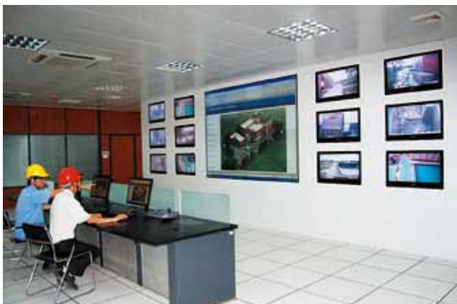
(1) Centralized control room for the transfer stations
