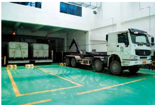
(2) Inside transfer station
