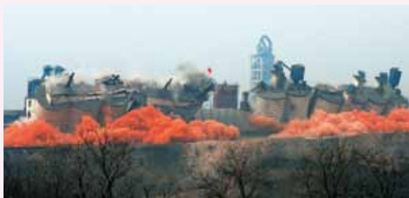
A cement plant in Shijiazhuang is blasted and demolished (Photo by Zhao Wei)
