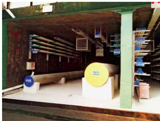
Figure 4-22 The utility tunnel in Pingtan comprehensive experimental area, Fujian (Photo by Liu Guangqi)
