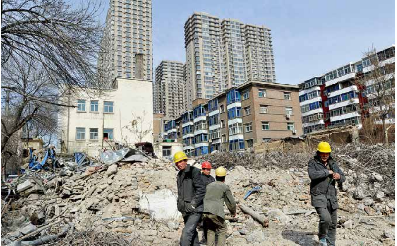
Figure 2-31 A village in Taiyuan City under demolition and renovation (Photo by Wei Liang)
