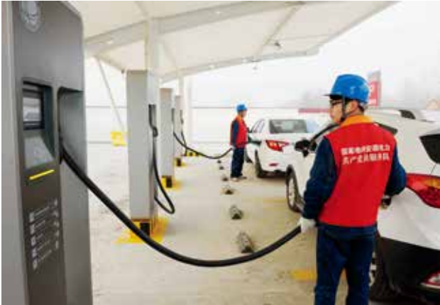
Figure 4-18 Charging stations for electric vehicles on Hefei-Xuzhou Expressway were fully completed (Photo by Song Weixing)
